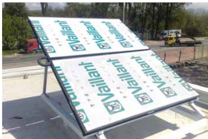
Sistem auroSTEP na pumpi Lukoil
